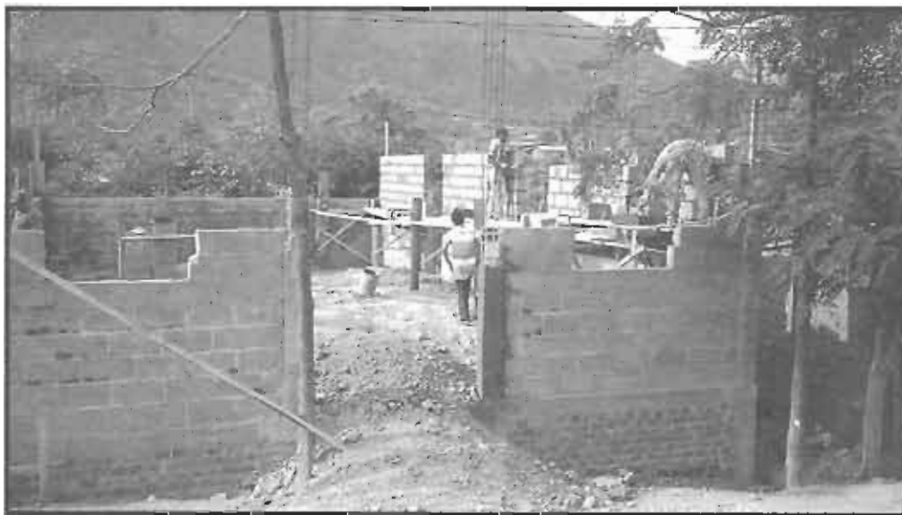
This is new church construction in Santa Ana, Ocotal, Nicaragua (made possible by Mrs. Becky Thompson in memory of her son). What a precious way to honor a loved one by giving a church to those who would never be able to have a church building.
