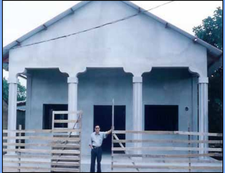
New Church Construction in Guaimaca, Honduras made possible by the Floyd Road Baptist Church in Austell, Georgia.
