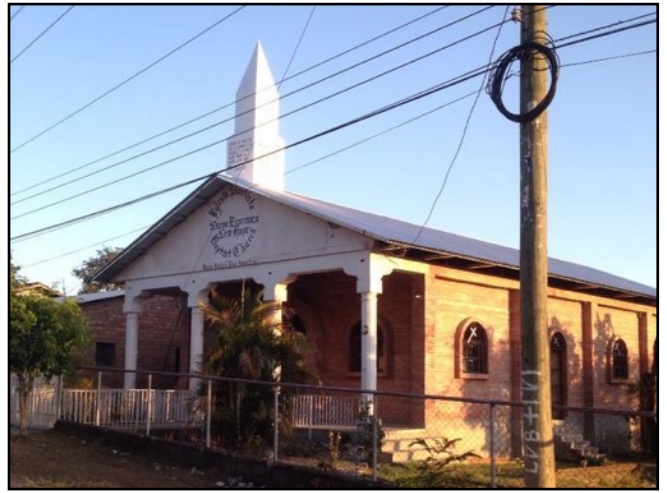
Church roof and steeple completed—We thank the Carpenters for Christ organization for giving the labor for this project
