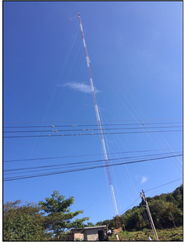
New 320 foot radio tower going up in San Marcos de Colon, Honduras
