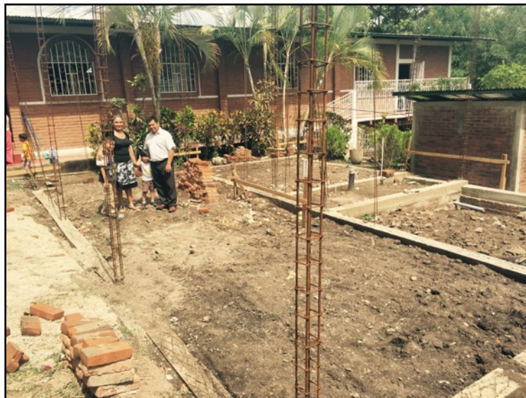
Pastor Santiago Urtecho and his family stand on what will be a new pastorium for his family so that the church will have more space for Sunday School rooms for the kids. We need help in finishing this pastorium in Yalaguina, Nicaragua.
